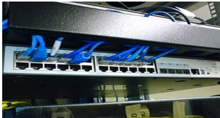
A rack mounted 24-port 3Com switch
